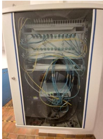
EDV Rack Trakt 1 UG
